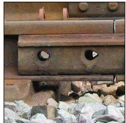
These bolt holes have been drilled incorrectly
