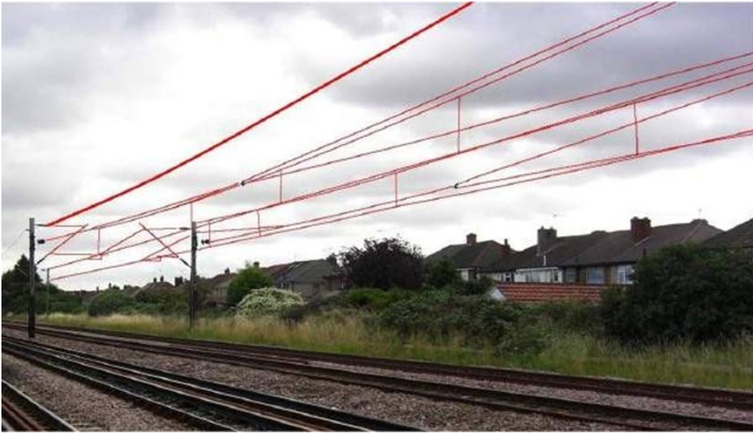
Example of Overhead Line Equipment
