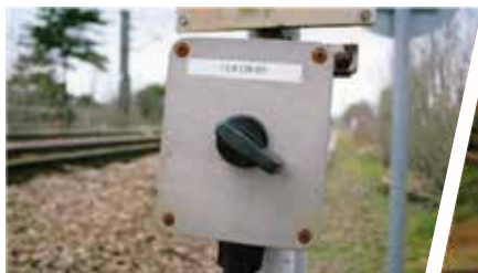
Example of a TOWS switch
