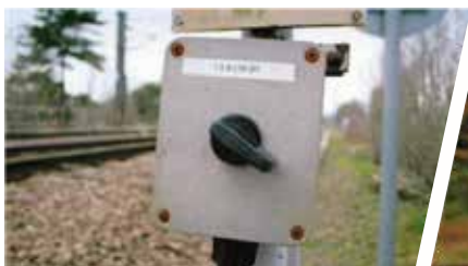
Example of a TOWS switch
