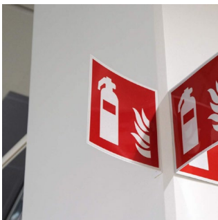
Fire equipment location - extinguishers
